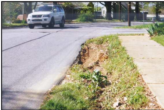
Located at the intersection of 7 th Avenue SW and 14 th Street SW, this ditch causes safety and appearance concerns.
