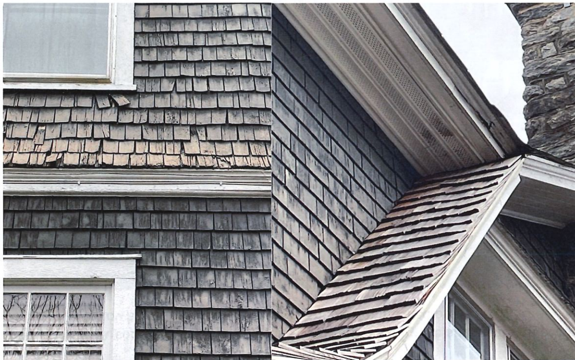
Figure 3: Applicant photo showing current siding conditions.
