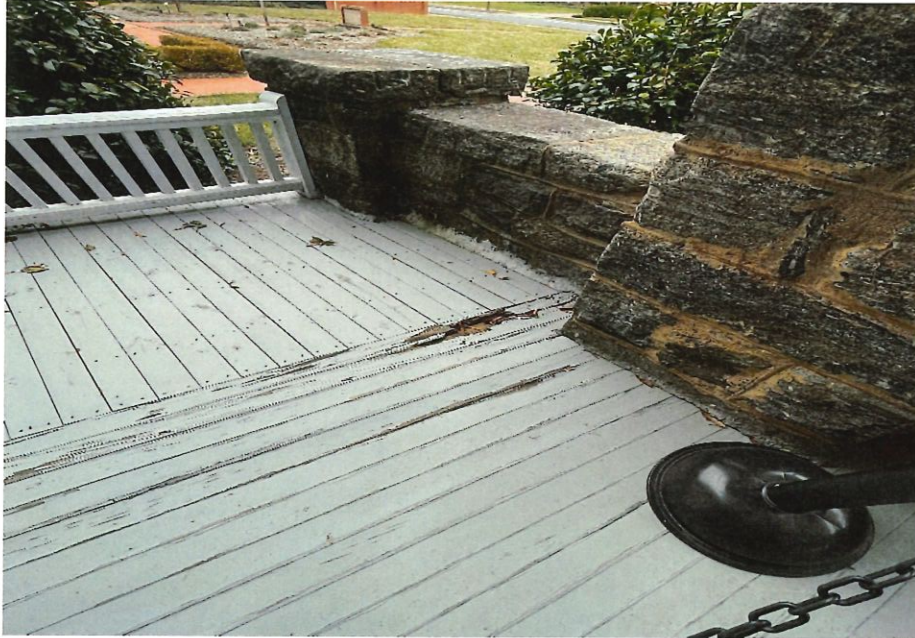
Figure 4: Applicant photo showing current porch conditions.
